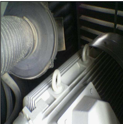
AIR INTAKE FILTER MOUTH NEAR MOTOR FINS
