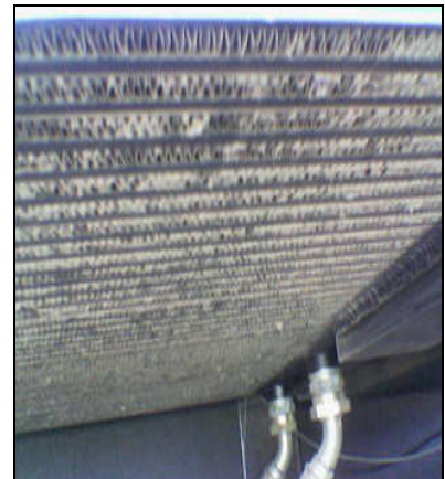
PARTLY CHOKED HEAT EXCHANGER in SKID
