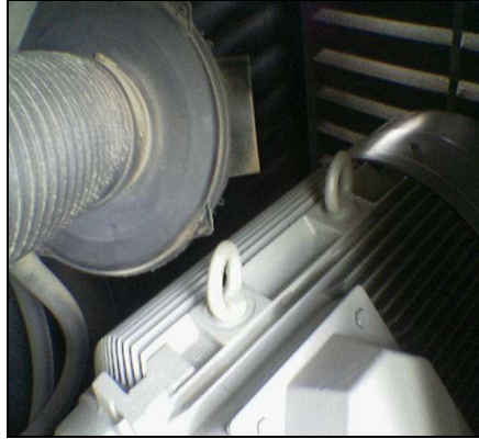
AIR INTAKE FILTER NEAR HOT ELEMENT & MOTOR
